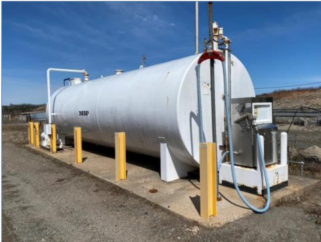
Figure 18-50: Diesel Fuel Farm
