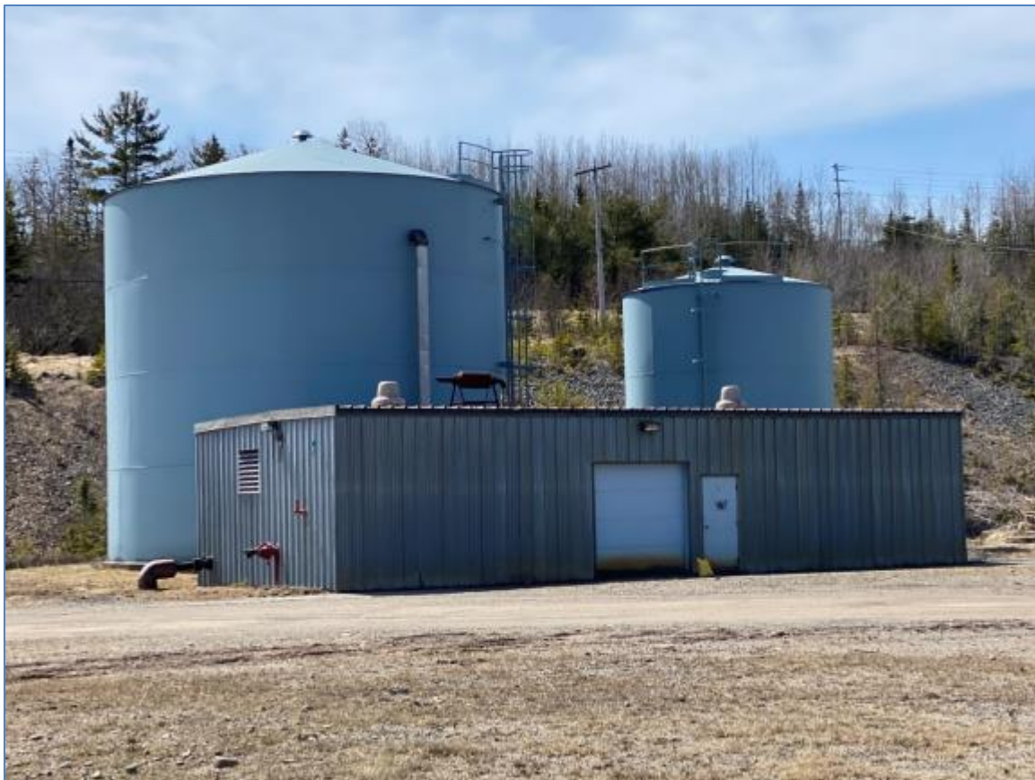
Figure 18-7: Water treatment plant and water storage
