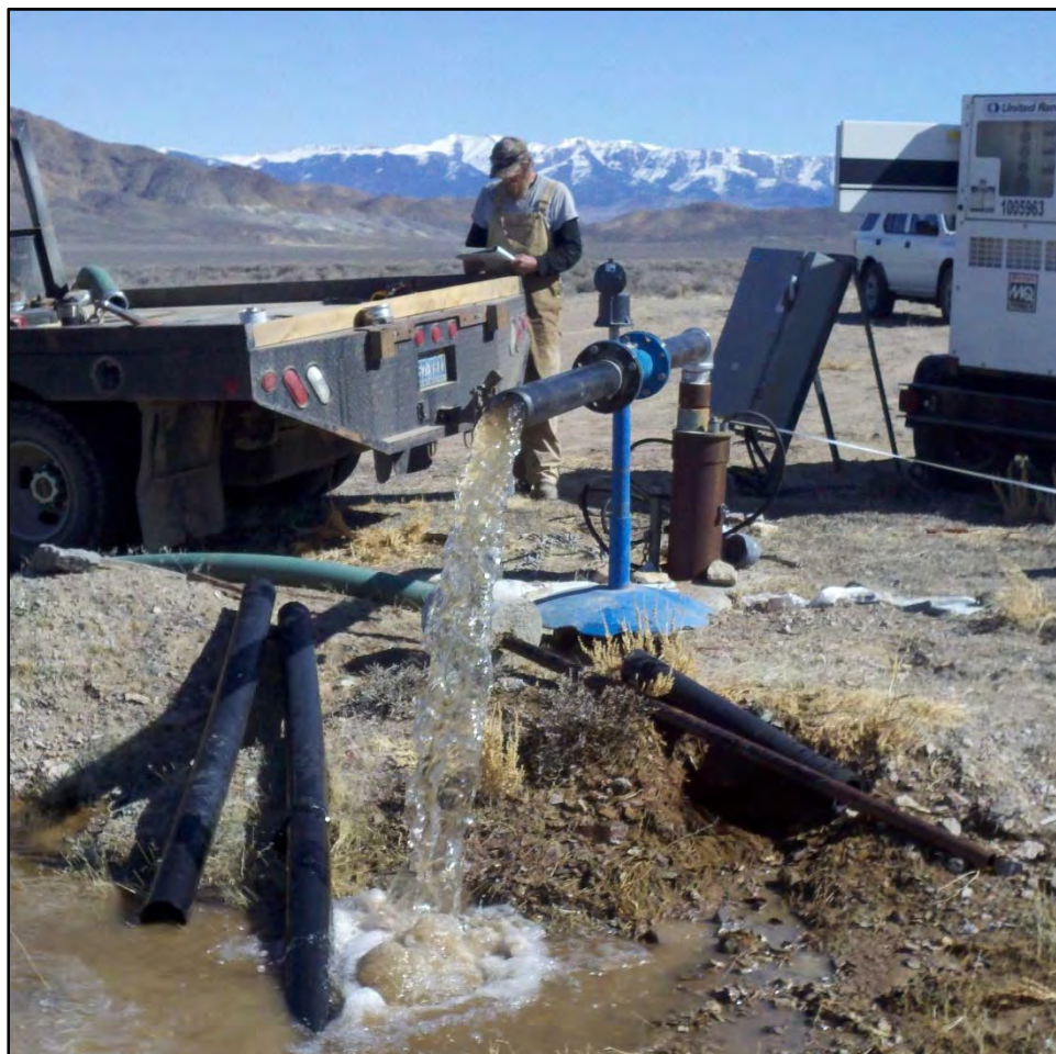
Figure 18.1: Photo of Water Well during Pump Testing
